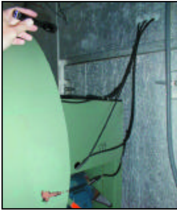
Figure 4 - Cables should be tied together so they cannot be damaged by rotating equipment, and should exit from the air handler unit in a centralized location.
