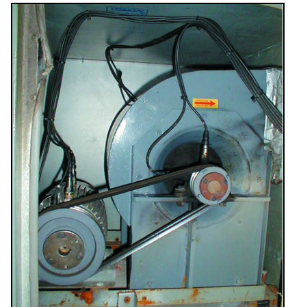
Figure 2 - The air handling units have fairly typical rotating elements, composed of two shafts supported by rolling element bearings, connected by a sheave-and-belt combination.
