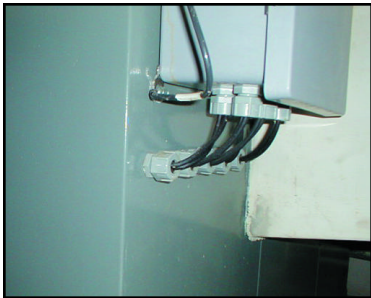
Figure 5 - One option used for this was to drill a hole in the side of the housing for installation of a cord grip and then seal it upon installation with silicone RTV.
